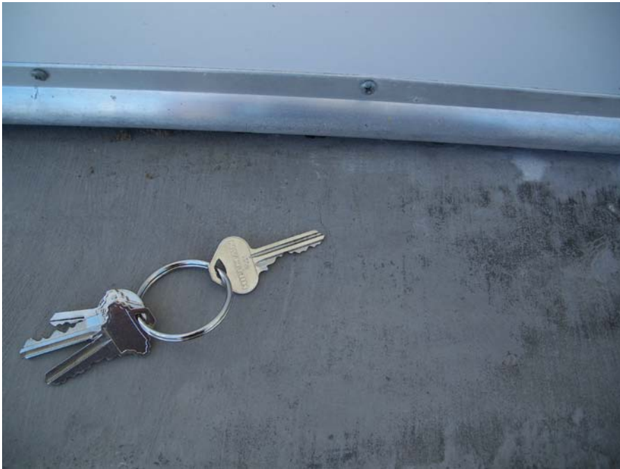
Photo #4 Patch Failure
