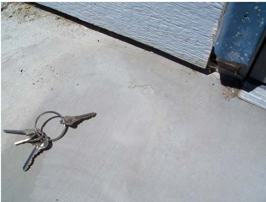
Photo #3 Patch Failure
