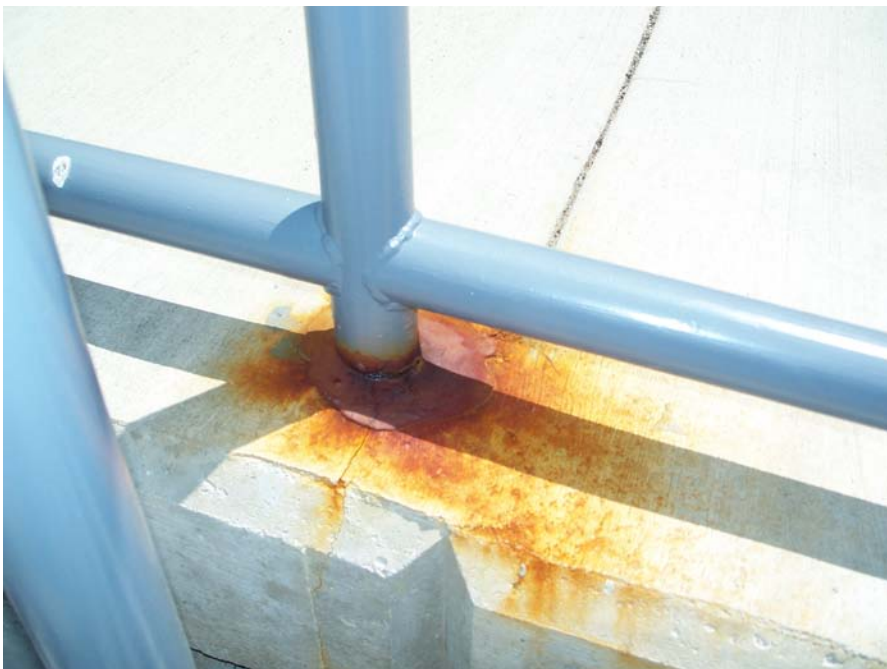
Photo #5 Handrail Rust
