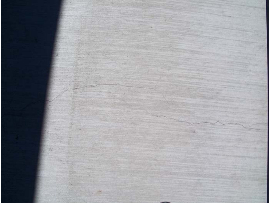
Photo #6 Increased Cracking
