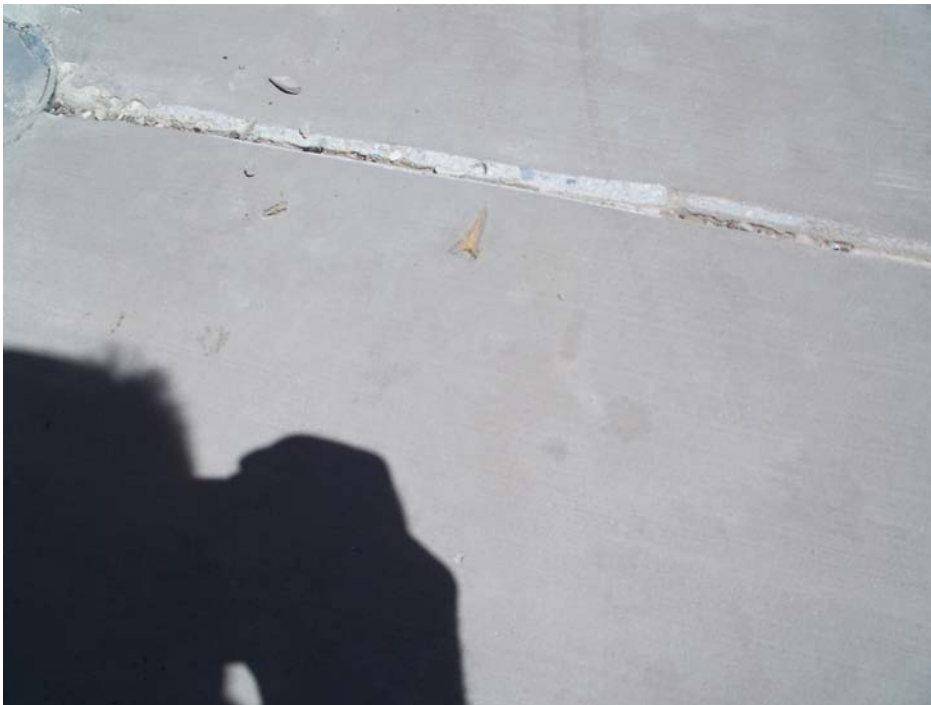
Photo #1 Patch Failure
