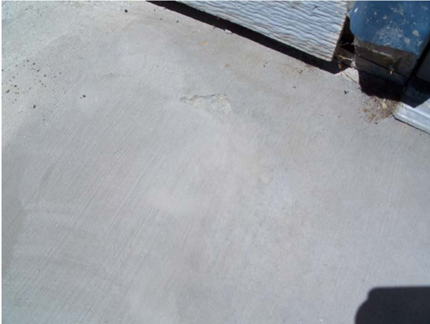
Photo #2 Patch Failure
